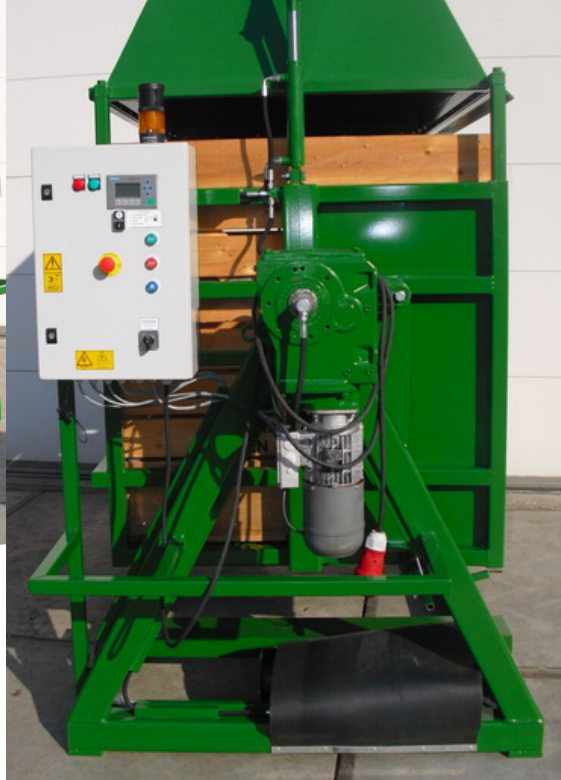
elektronic motor and control box
